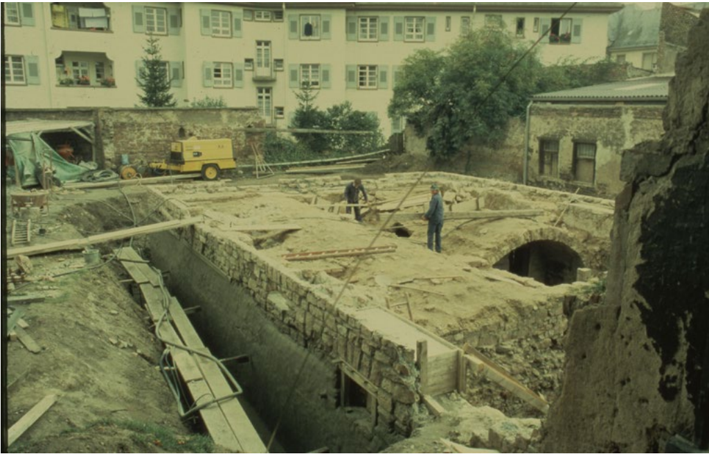
Fig. 13: Vaulted cellar which have been preserved from the former community hall, c.1979/1980
