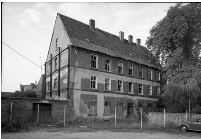
Fig. 30: The former Old People's Home of the Jewish Community Worms, in dilapidated state. Historical photograph, September 1970
