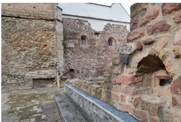
Fig. 5: Listening window (right) and remains of the seating bench with reconstructed covering (below) in the women's shul in Speyer Jewry-Court , current state
