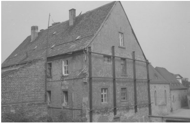
Fig. 28: The former Old People's Home of the Jewish Community Worms, in dilapidated state. Historical photograph, August 1969
