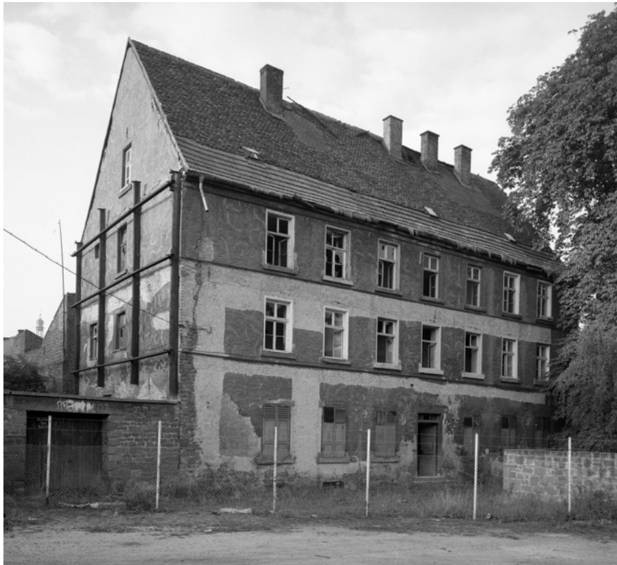
Fig. 9: The former Old People's Home of the Jewish Community Worms, in dilapidated state. Historical photograph, September 1970
