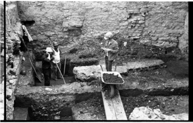
Fig. 33: Excavation of the medieval cellars of the former community hall before the building of today's Rashi House . Historical photograph, 1980
